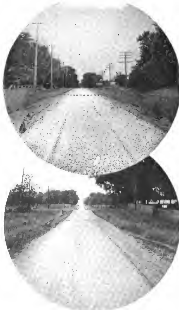
Upper—A finished macadam highway adjoining a loose stone roadway that has the material merely thrown on with a shovel. The soil underneath has been well crowned and side ditched, but no side retaining earth curb has been cut to hold the stone. Lower—A stone road recently resurfaced. Traffic has done most of the rolling to bind the stone. One rut starting to develop on right side
